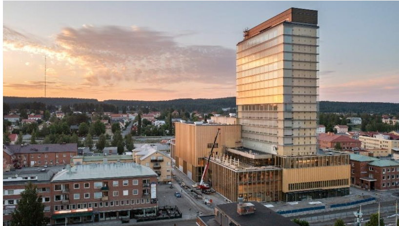
Figure 26: Birdview of the Sara Kulturhus Centre in Skellefteå. Photo by Åke Eson Lindman
